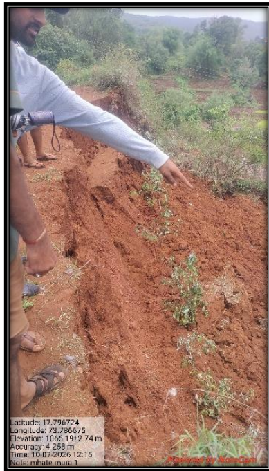
Photograph No.5 Picture showing Downslope Mass Creep
