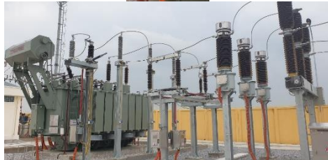
Fig.3 A real voltage tap changer of a three-winding transformer
